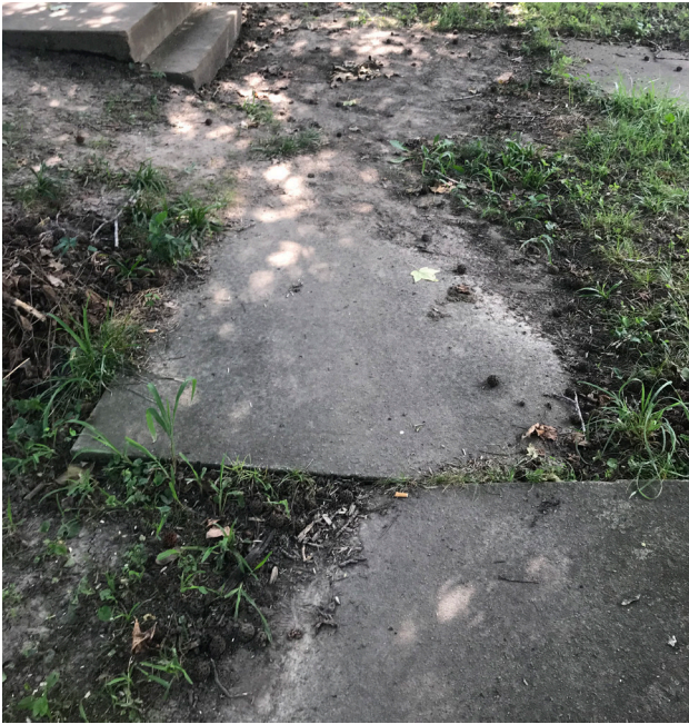
Sidewalk in poor condition on a local street.
