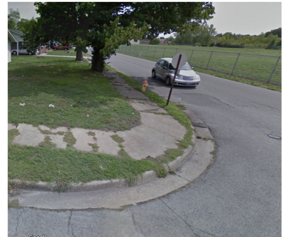
NO CURB RAMP
